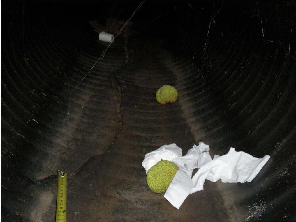
Photo3: Longitudinal crack along pipe flow line (east end, south pipe)
