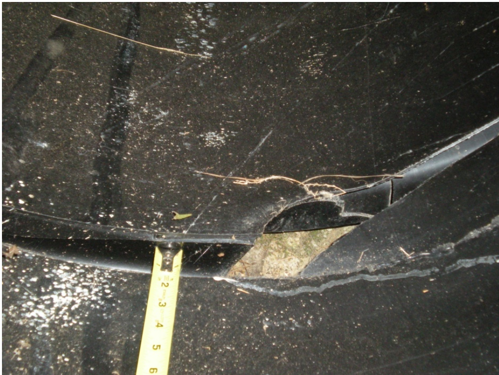
Photo2: Separation and crack of two joints of pipe (east end, north pipe)
