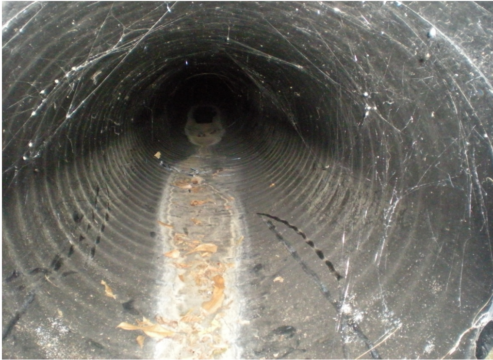
Photo 5: Area of pipe of transverse cracking and failure. (north pipe, east end)
