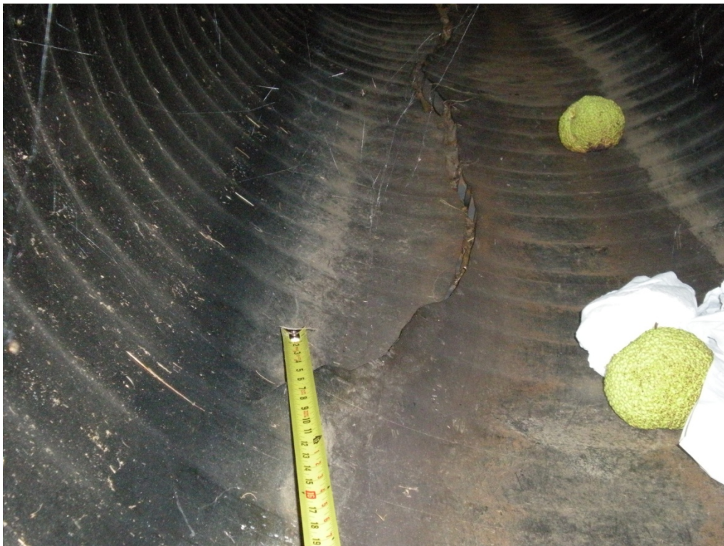
Photo 4: Closer view of longitudinal crack. Right side of pipe beginning to elevate
