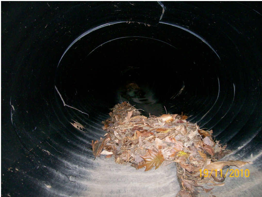
Photo 6: Transverse cracking and failure near joint. (south pipe, inlet 1, west-facing)
