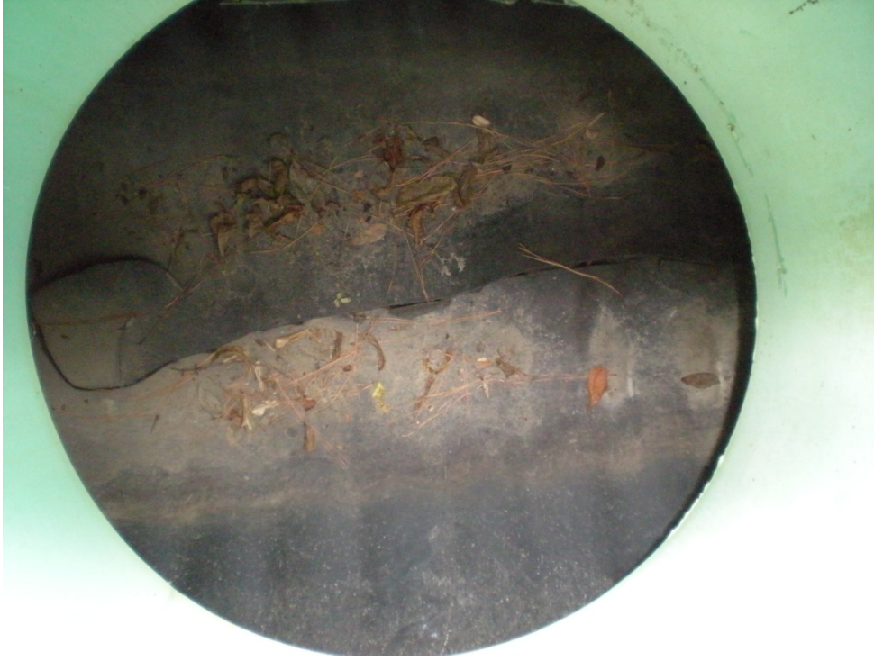
Photo1: View of crack in bottom of pipe at Inlet #1.
