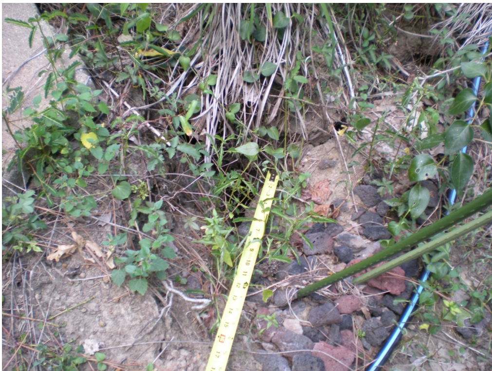
Photo 8: View of sinkhole developing above the existing pipe
