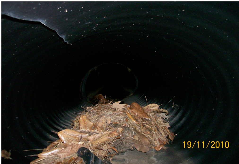
Photo 7: Longitudinal cracking in top of pipe. (south pipe, inlet 1, east-facing)
