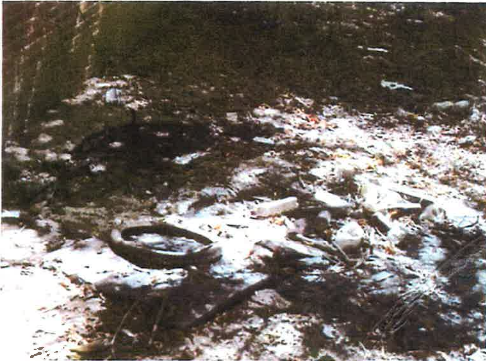
Open cleanout behind building
