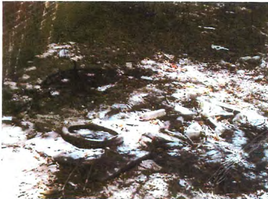
Open cleanout behind building
