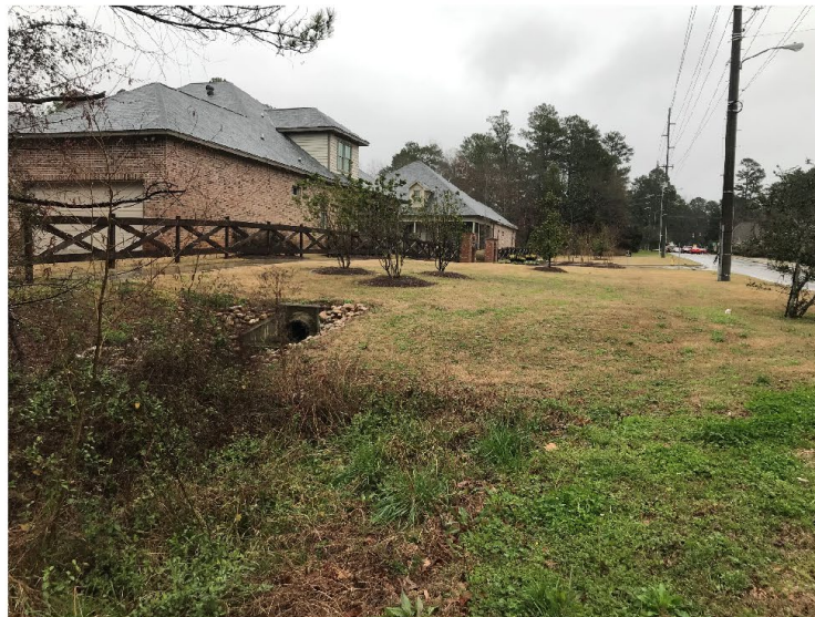
Photo Location 2 – Looking east at drainage pipe within ROW at Riddle Run's southwest corner.
