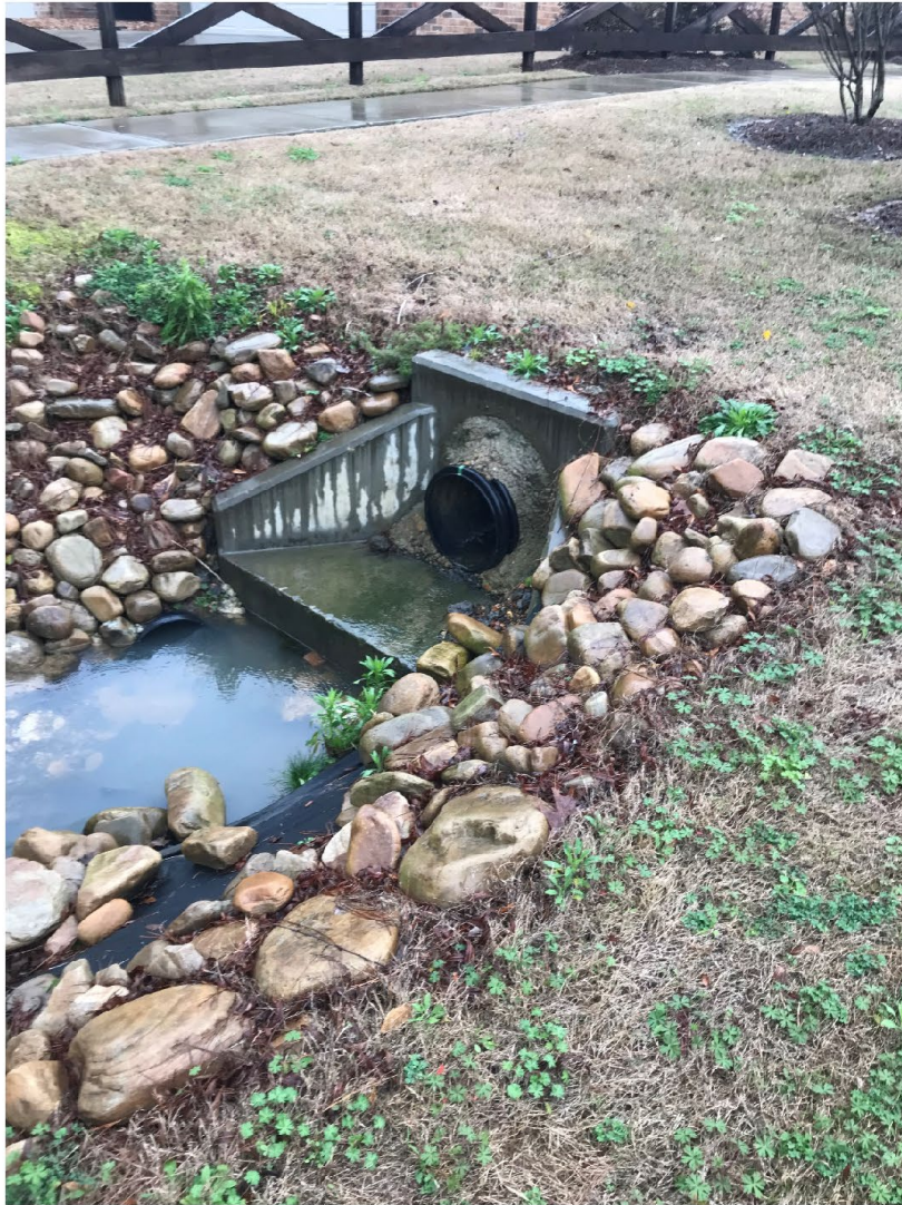
Photo Location 2 – drainage pipe discharging within ROW at Riddle Run's southwest corner.
