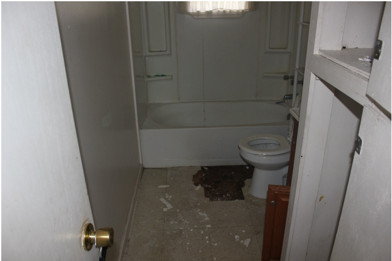
Bathroom floor tiles missing and soft floor from water damage.
