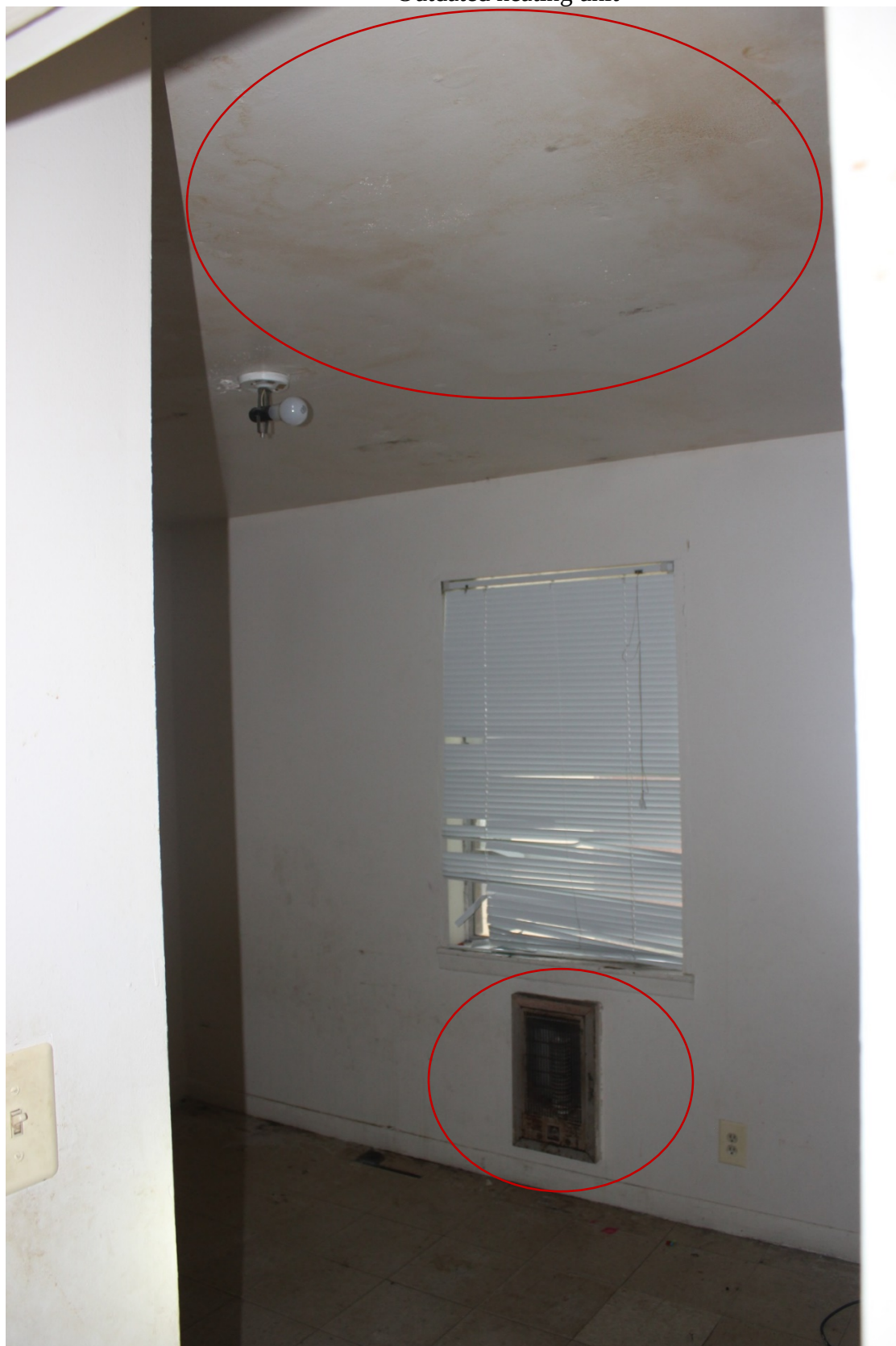
Discolored spots in ceiling Outdated heating unit
