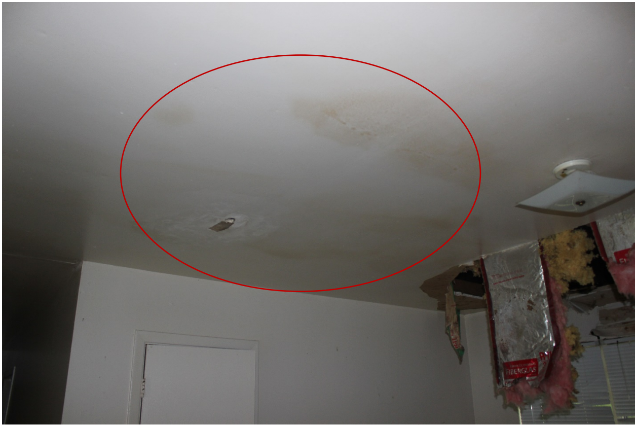
Discolored spots in ceiling from water damage
