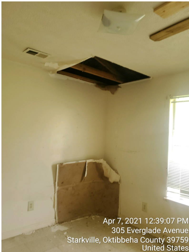
Large hole in back corner of the room.
