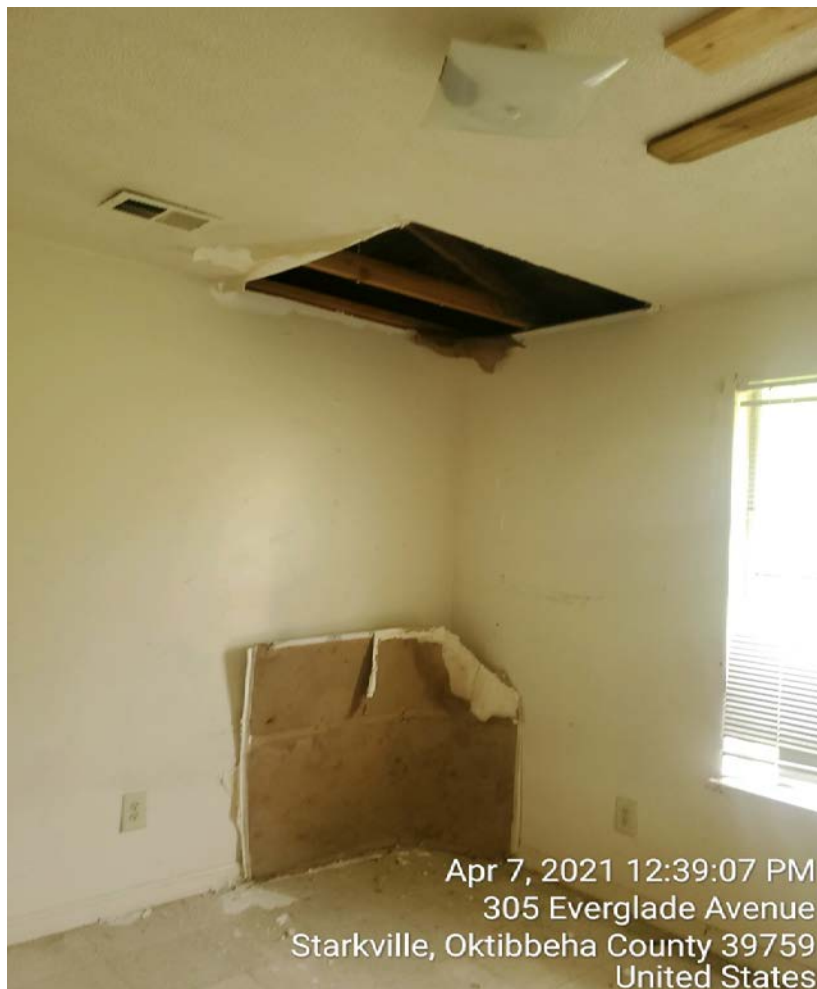
Large hole in back corner of room.
