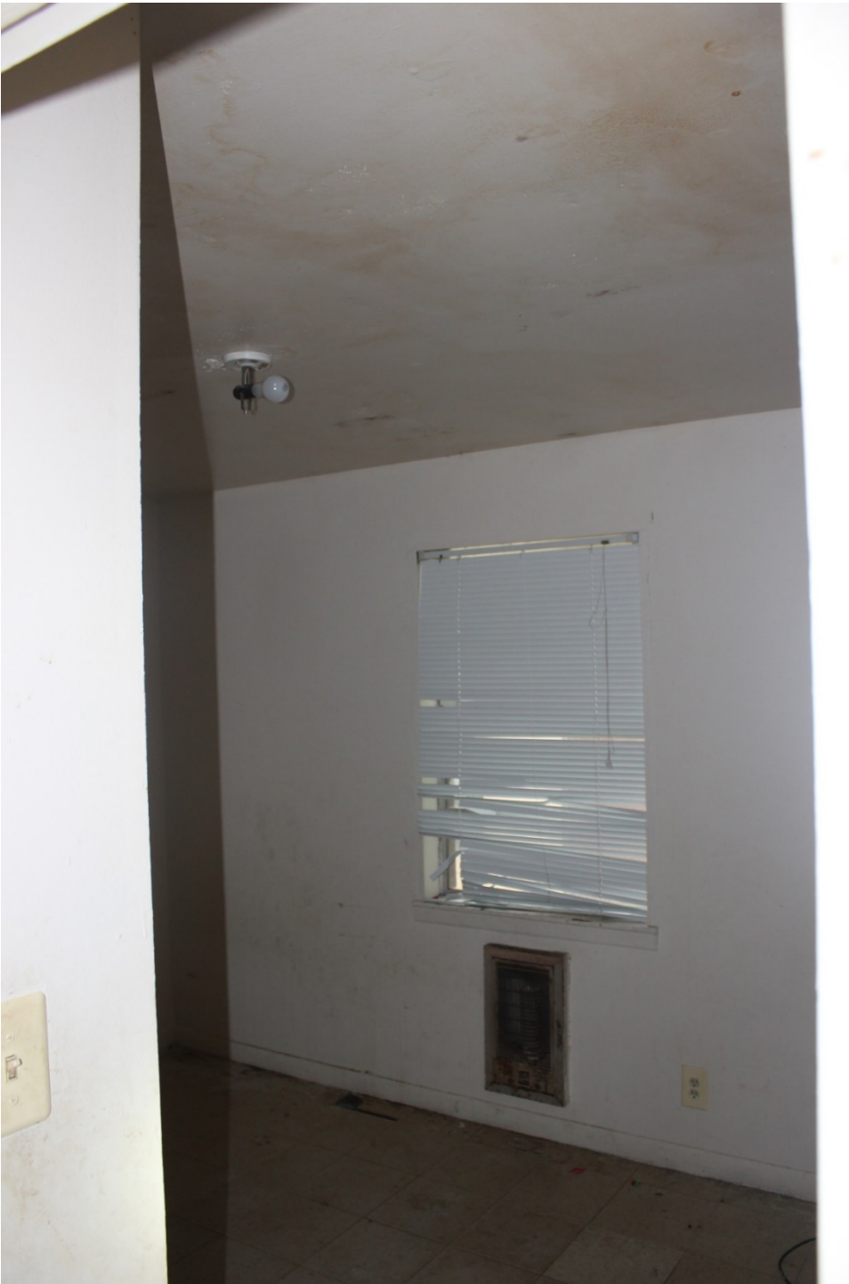
Discolored spots in ceiling - Outdated heating unit
