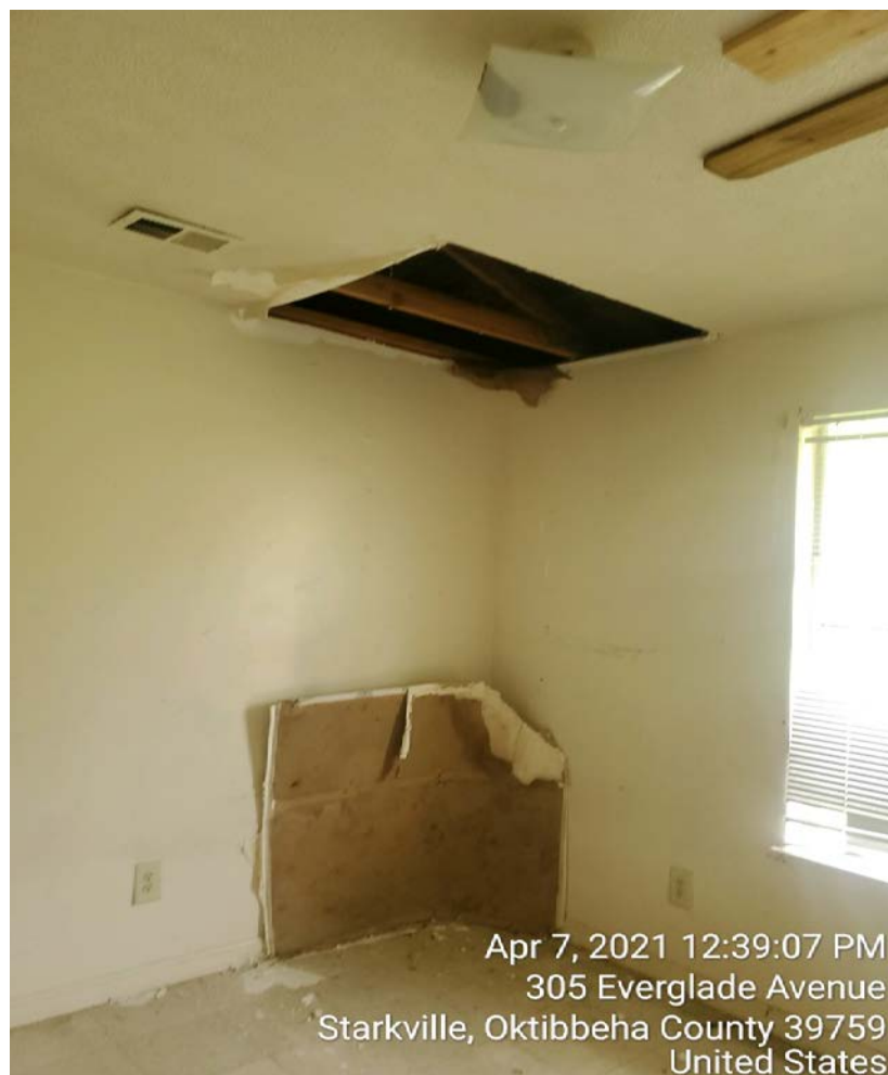
Large hole in back corner of room.
