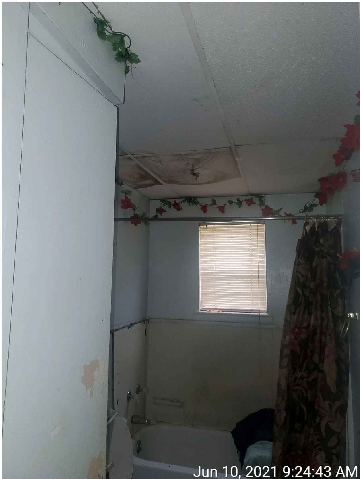
Unit B Bathroom has damage to the ceiling
