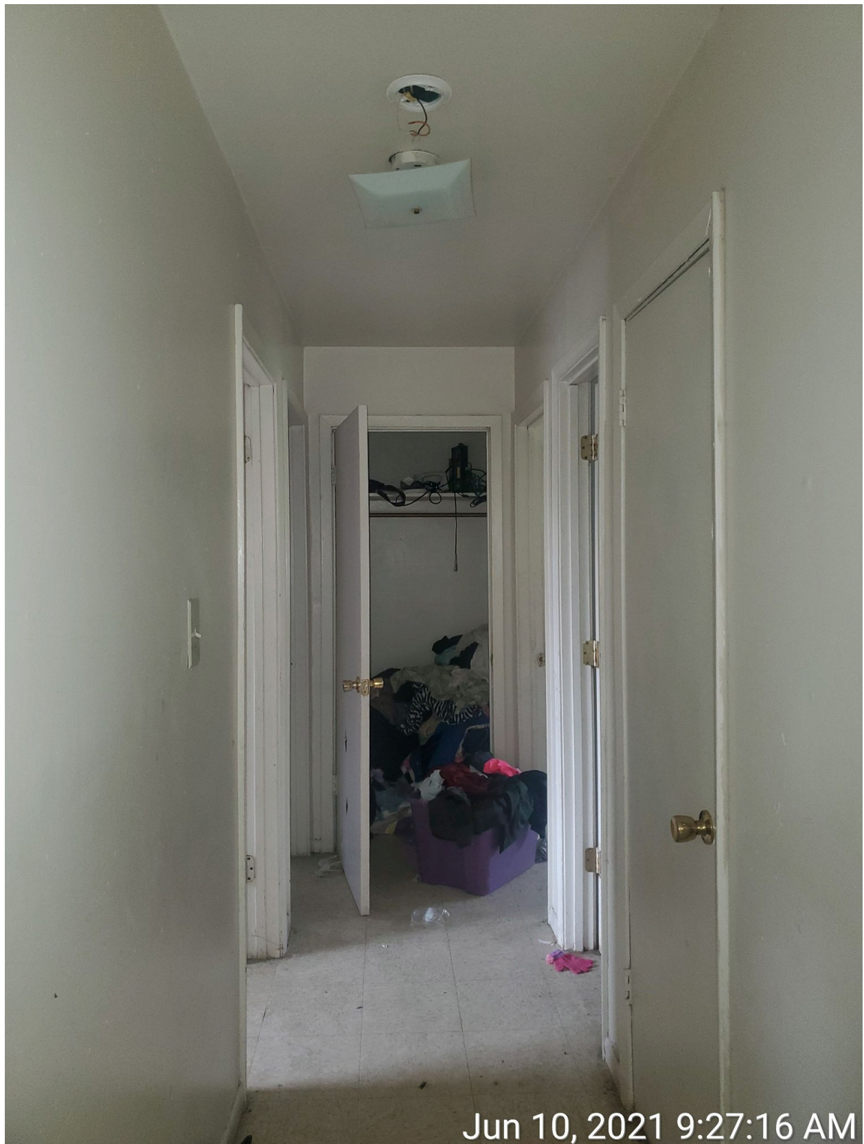
Hallway smoke detector missing
