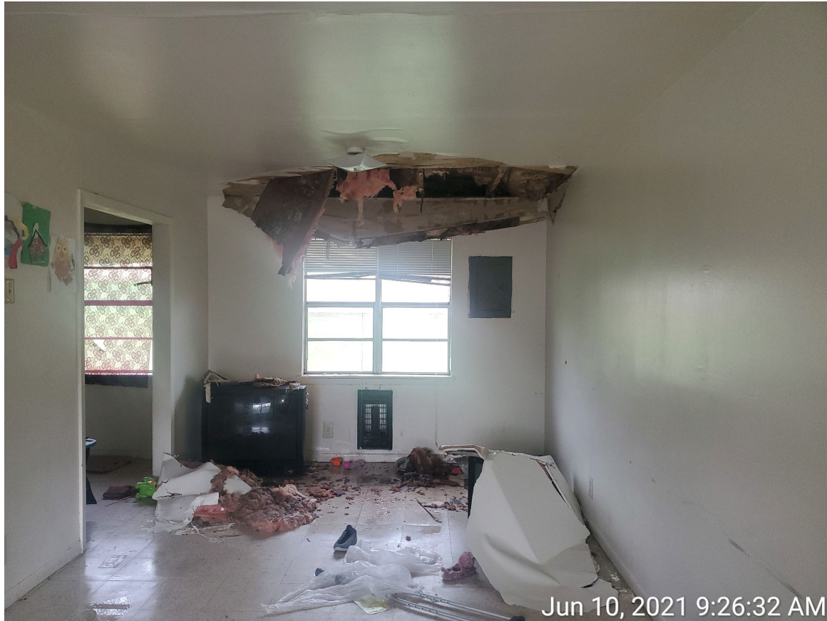
Unit C unoccupied Dining area ceiling collapsed floor soaked through and very weak.
