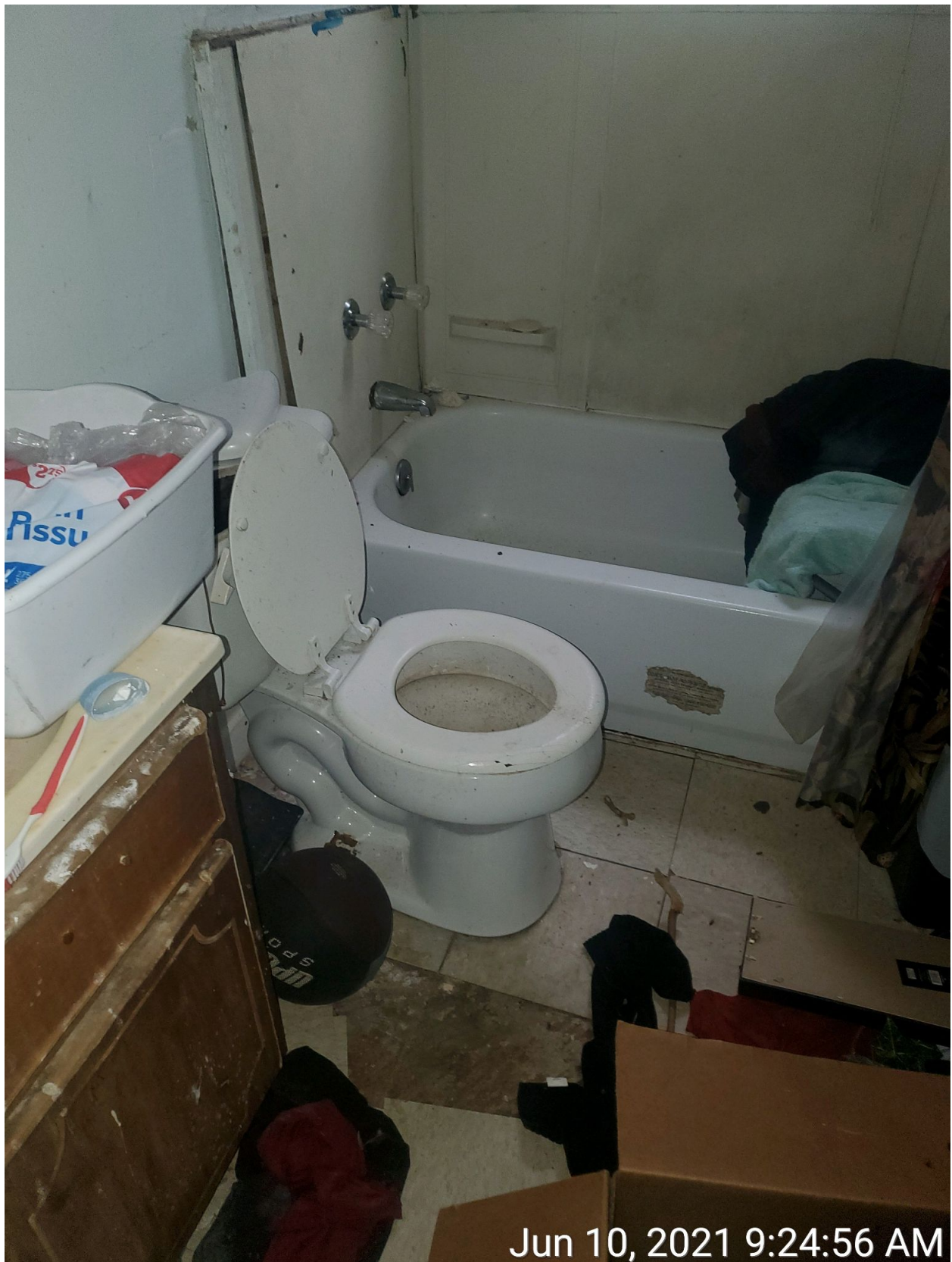
Missing floor tiles
