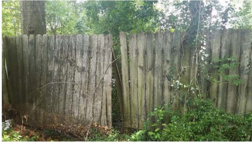
Figure 4: Example of Splitting and Warping Fence along Property Line in Back Yard
