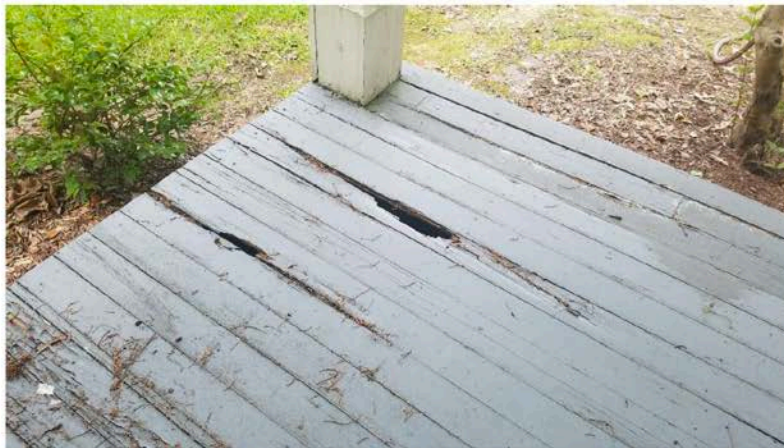
Figure 10: Rot Damage in Porch Floorboards
