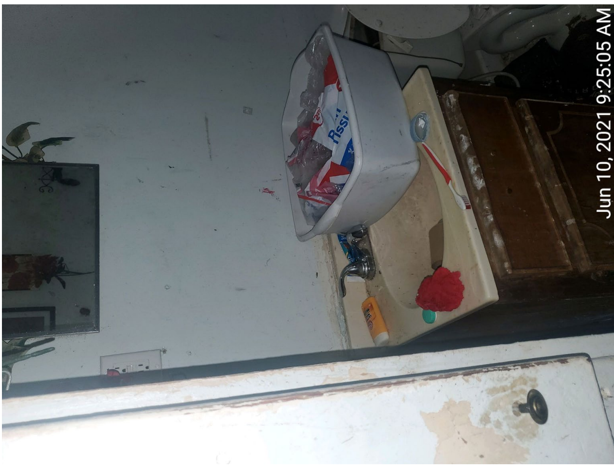
Building # 10 Apartment B Bathroom there is more left behind belongings and missing tiles from the floor.
