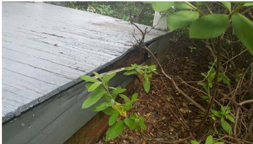
Figure 12: Detail of Damage to Fascia and Buckling of Boards
