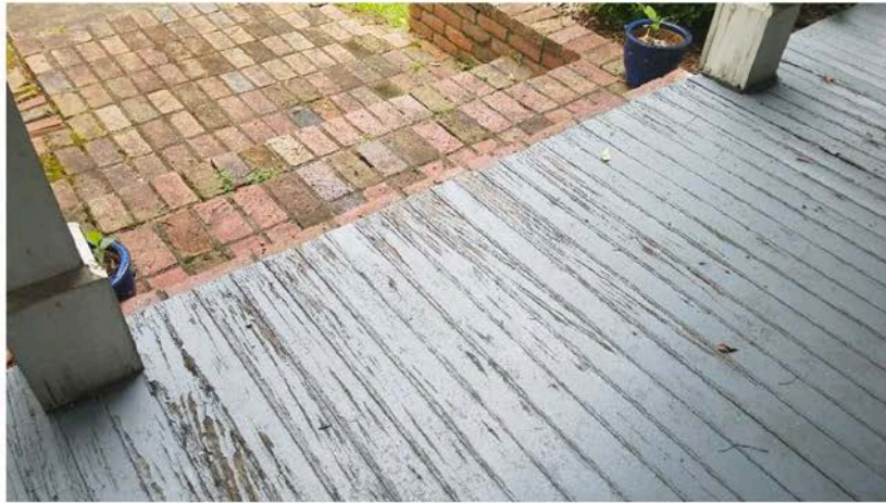
Figure 11: Buckling of Porch Floorboards in Entry
