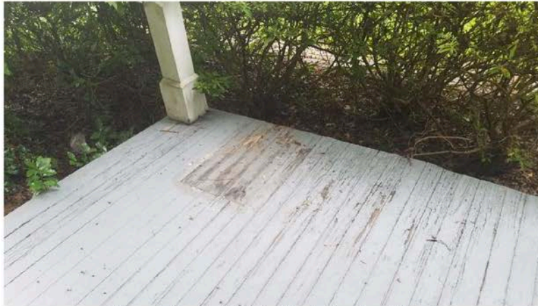
Figure 9: Detail of Existing Porch Floorboard Repair
