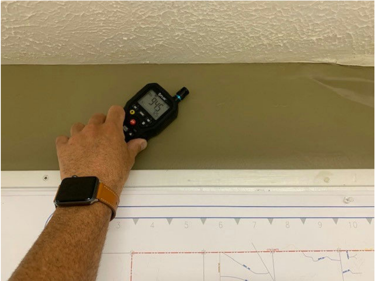
11 11-FD break room moisture reading
