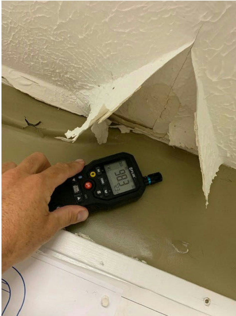
10 10-FD moisture reading in drywall from roof leak
