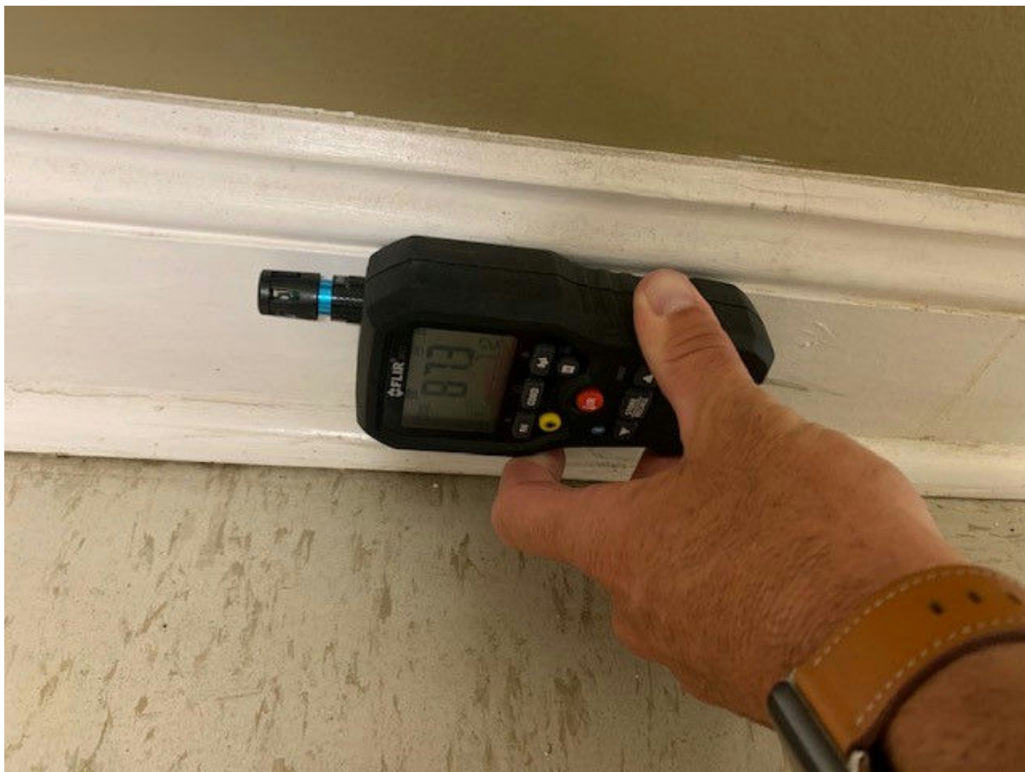
12 12-FD base board moisture reading
