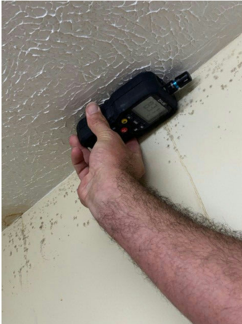
3 3-FD moisture reading on ceiling in stairway
