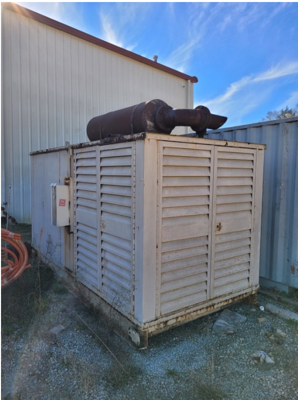
Electric Division Diesel Generator Not in working condition
