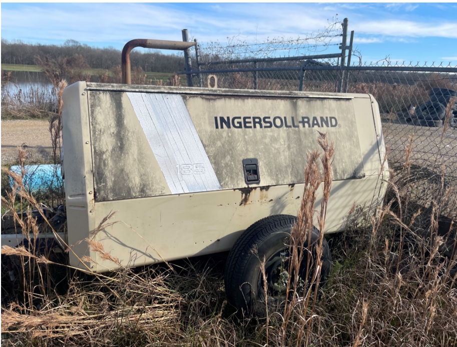
Water division older Generator
