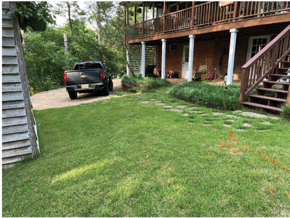
Figure 3. Rear entry into the partial basement from the west side of 227 Lakewood. Note the tail end of the retaining wall on the northwest corner of the home - the approximate location of 1965 amendments to stabilize the subsiding corner of the home. This corner of the home, between the house and shed, is not suitable for construction due to the elevation change, soil instability, numerous buried underground utilities, and proximity to mature oak trees.
