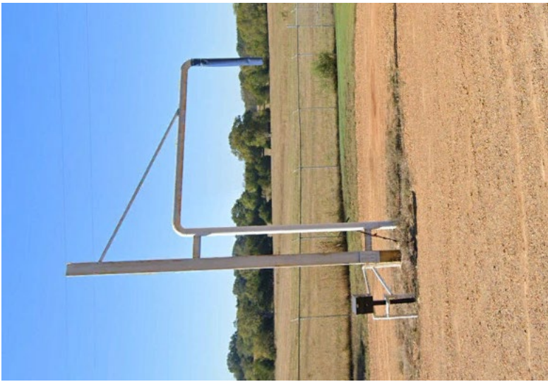
Portable Tank Filling Station
