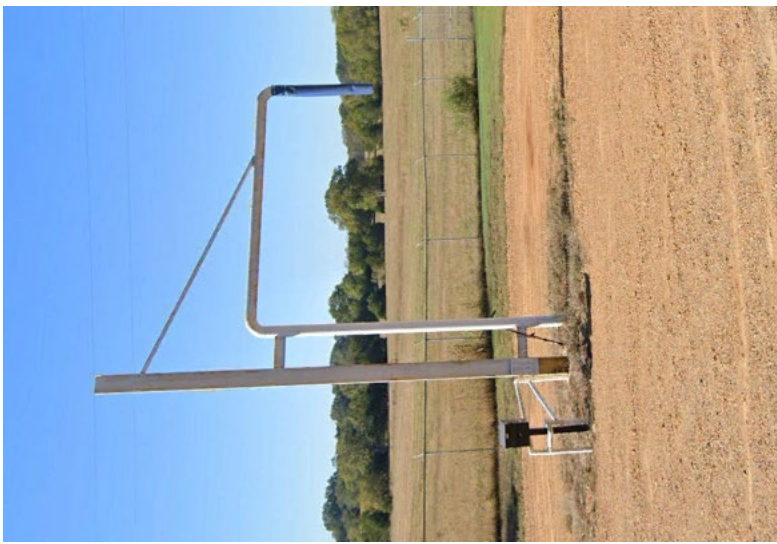
Portable Tank Filling Station
