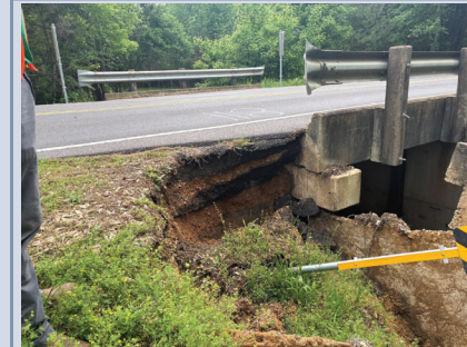
ROADWAY UNDERMINED SEVERE SHOULDER EROSION
