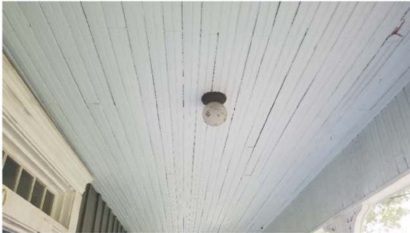
Figure 13: Existing Light Fixture
