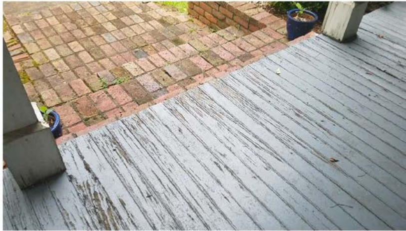
Figure 11: Buckling of Porch Floorboards in Entry
