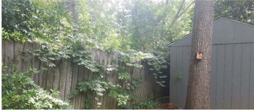
Figure 7: Buckling of Fence Along Neighboring Property
