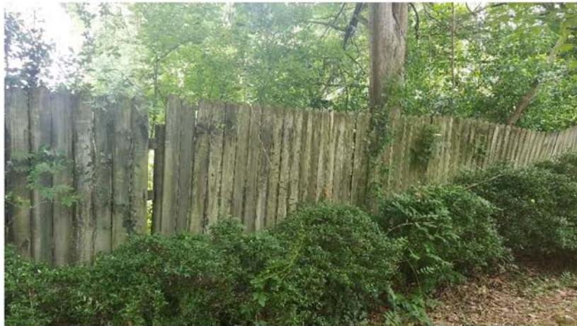
Figure 5: Additional Example of Splitting and Warping Fence along Property Line in Back Yard
