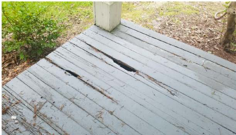
Figure 10: Rot Damage in Porch Floorboards
