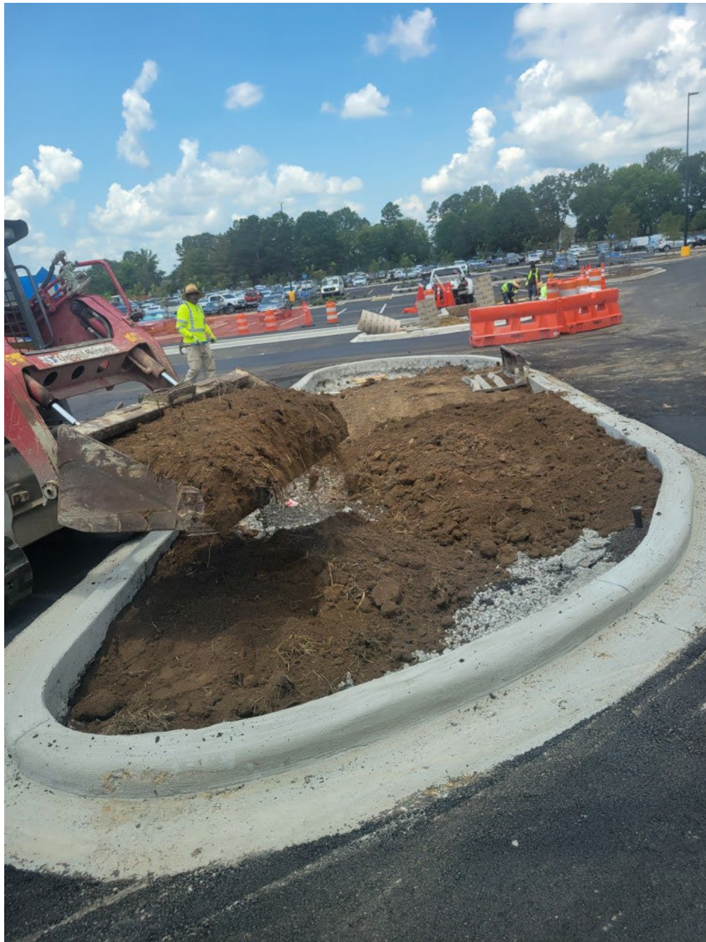
While onsite, the contractor was also observed placing topsoil or plant mix on top of compacted subbase material.
