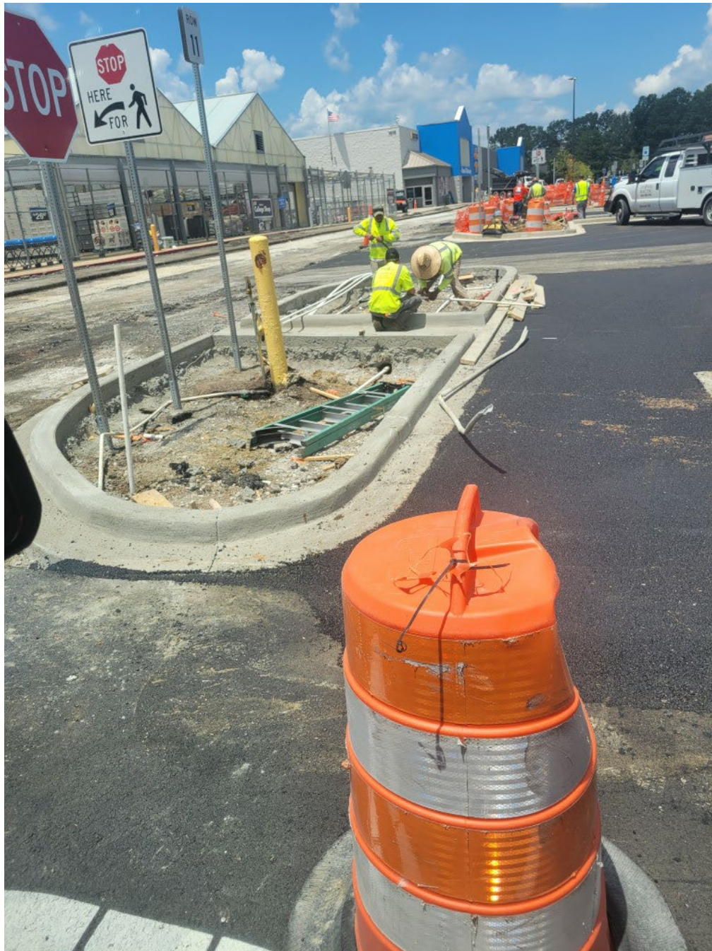
Irrigation is being installed in a landscape island. The subbase material has not been removed.
