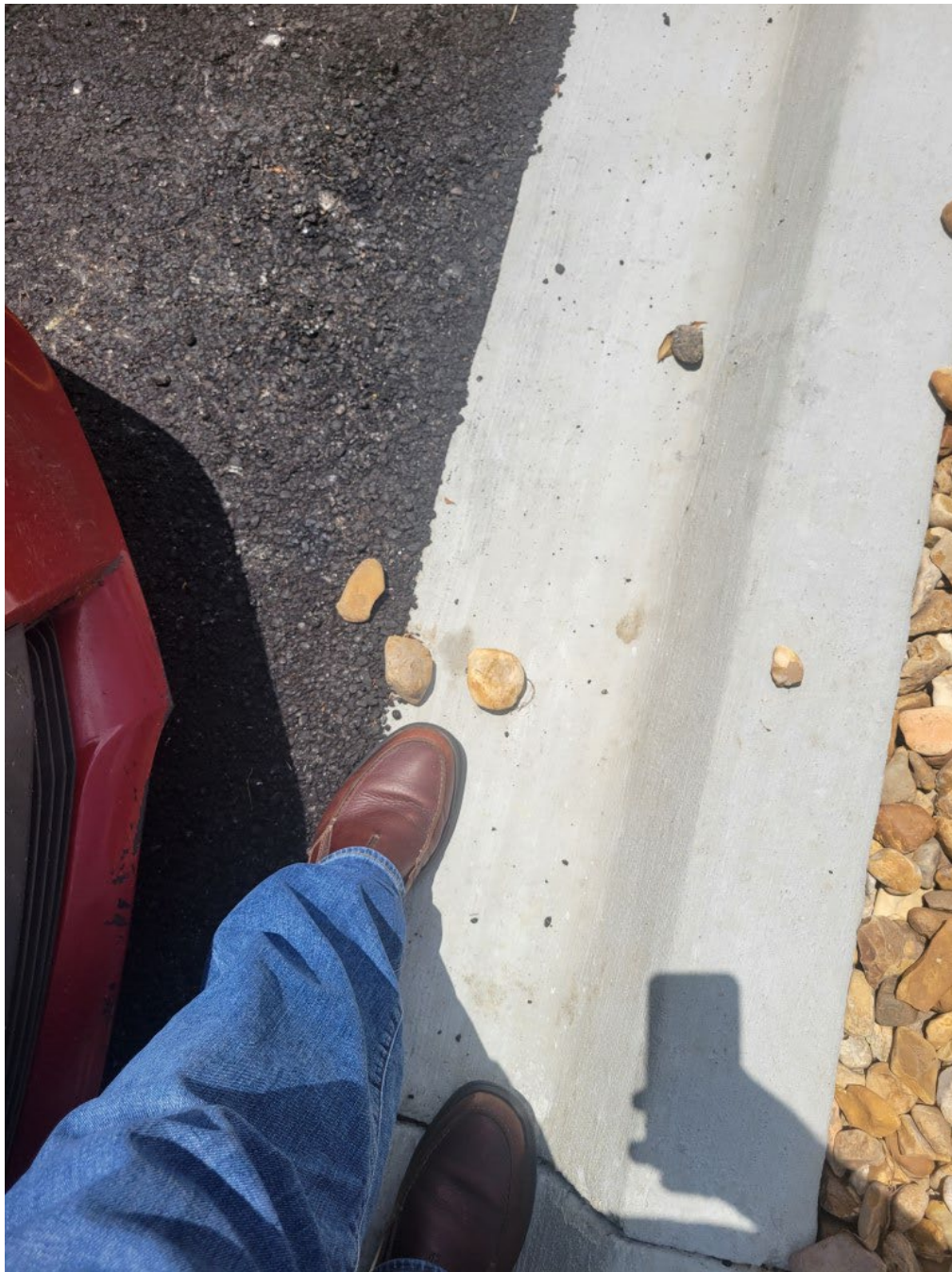
Rocks present a tripping hazard
